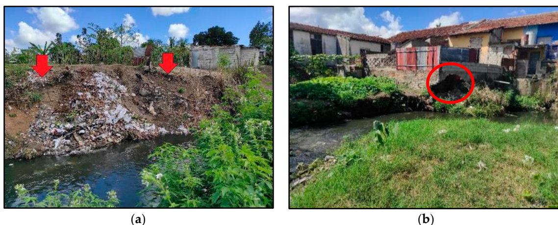
Figure 8. (a) Water footprint observed in the field after the occurrence of a severe hydrometeorological storm, 25–26 May 2020 [11], and (b) photograph of the damage to structures near the Cubanicy riverbed.
