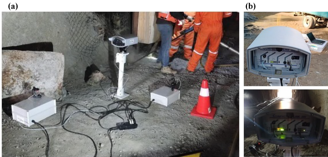
Fig. 4 a Installation of the communication system in the mine, b FSO transceiver within the mine tunnel, top: outside the tunnel, below: inside the tunnel
